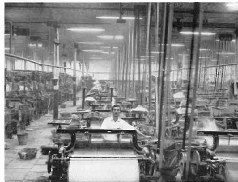
Problems involved in the detailed job of weaving are simplified by the introduction of fluorescent lighting at Shree Niwas Cotton Mills, Bombay.
