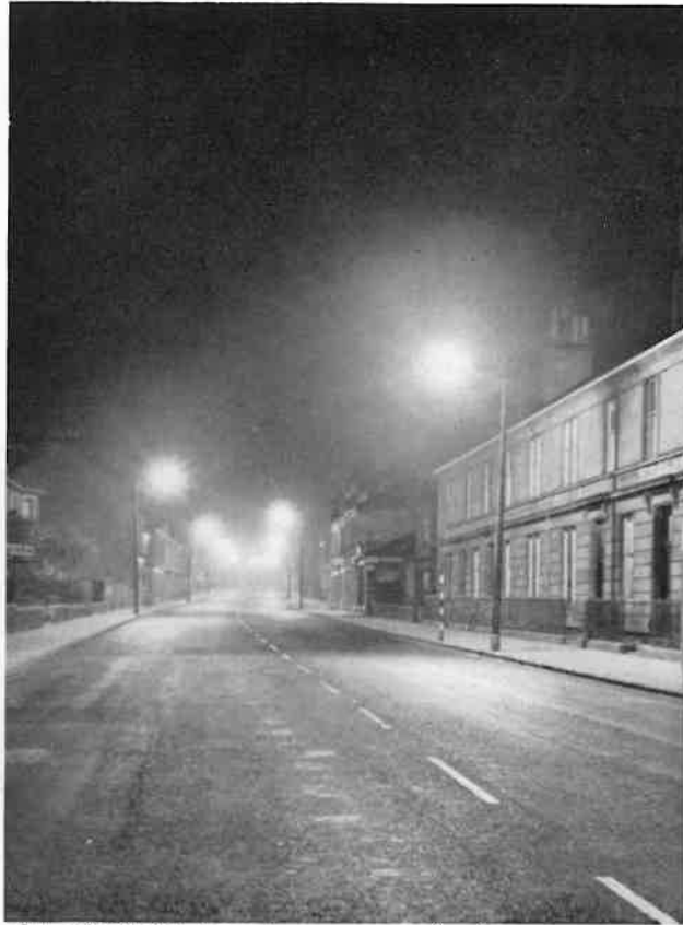
One of Britain's largest installations of sodium vapour street-lighting, on the Glasgow-Carlisle Road. Lamps are 140 watt in enclosed type lanterns. Mounting height 26 ft. spacing 120 ft.
